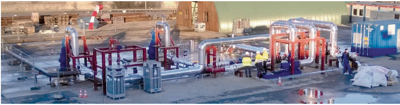
View of the well site with the two wellheads on the left side.
